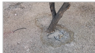
Irrigation emitters left too close to trunk; one not working
