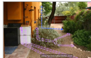
Combined graywater and rooftop rainwater harvesting. Photo credit: HarvestingRainwater.com
